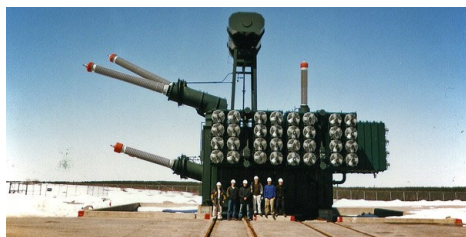
A Hydro-Quebec HVDC converter
